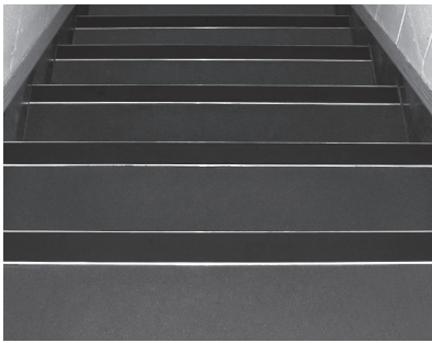
Partially-sighted People Poor Tonal Contrast Picture 2
