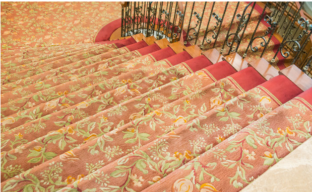
✗ Critical surface: Patterned carpet and no stair edgings - staircase looks like a ramp
